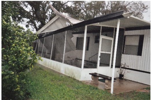
Lot 19's roof getting ripped off
